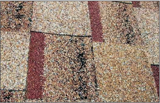
Manufacturing Defects – This may occur during the manufacturing of shingles.
